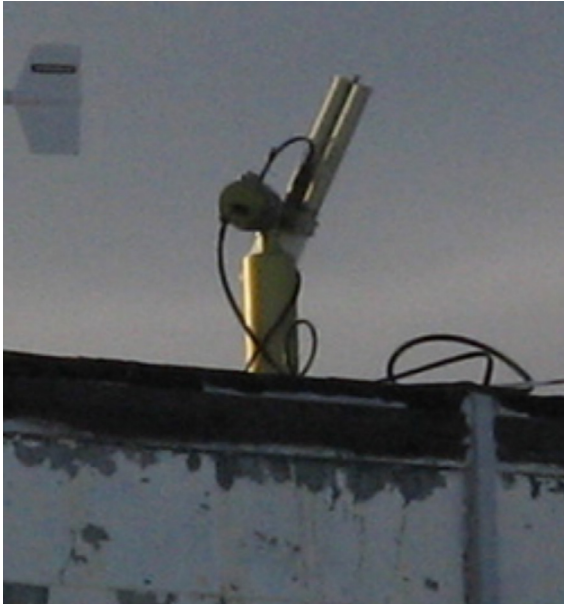
Figure 5. The Cimel installed on the roof of building #1985.
